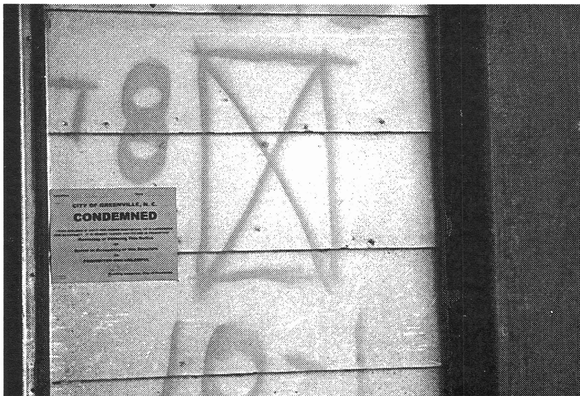
Approximately 6000 structures in Eastern North Carolina were condemned following the flooding of Hurricane Floyd (photo by Katherine Jones).
